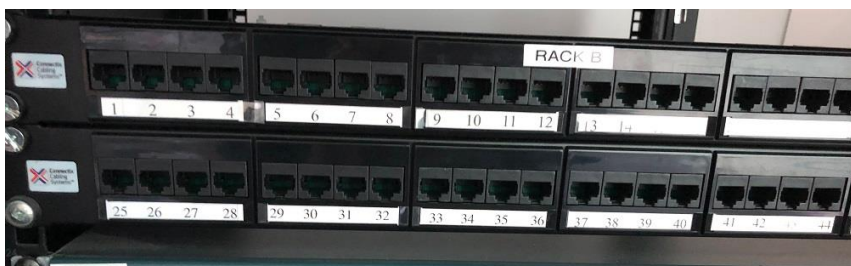
Figure 3: The patch panel (one of 2 panels in CM142)
